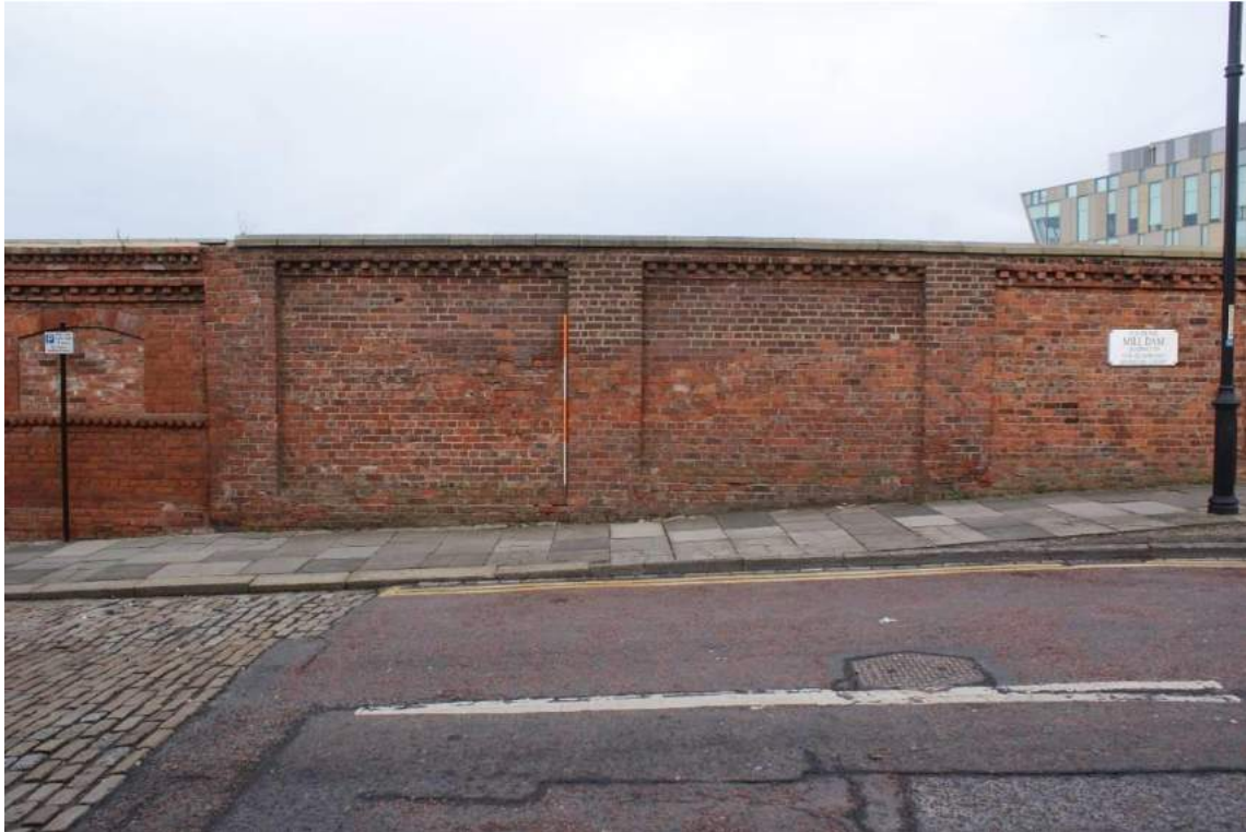
Plate 27 Wall Sections (D1 and D2), showing rebuilding to top of wall, looking north-west
